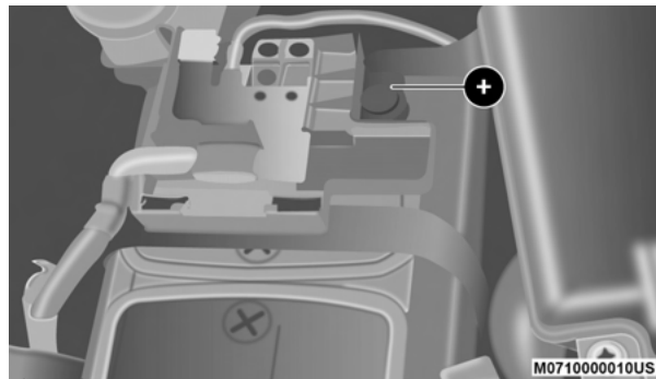
Positive Battery Post Location
